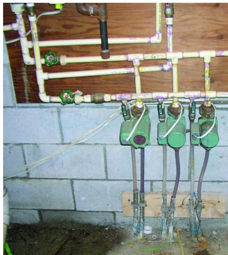
Figure 2. Radiant Distribution Manifold and Circulators
