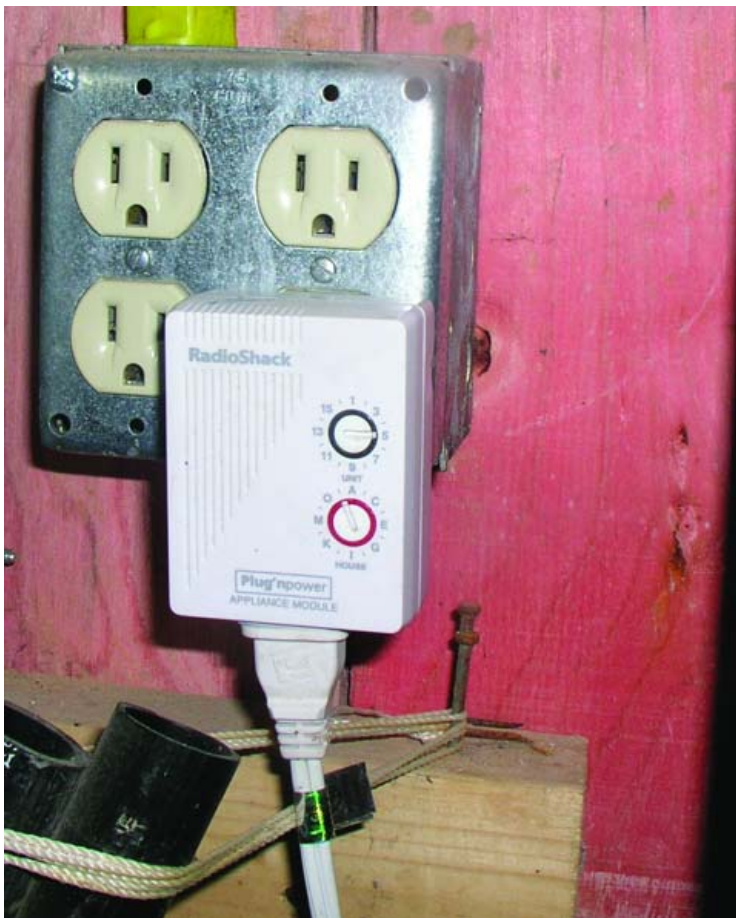
Figure 3. Radio Shack/X10 Appliance Module Controlling Circulator
